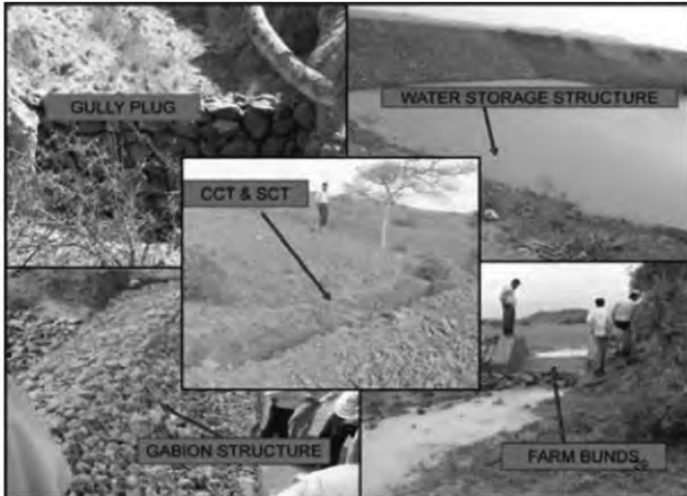
Rain Water Harvesting Structures
