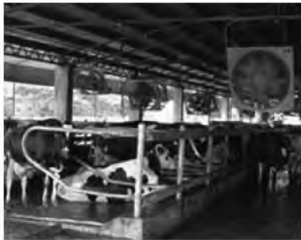
A typical Fans and spray arrangement
